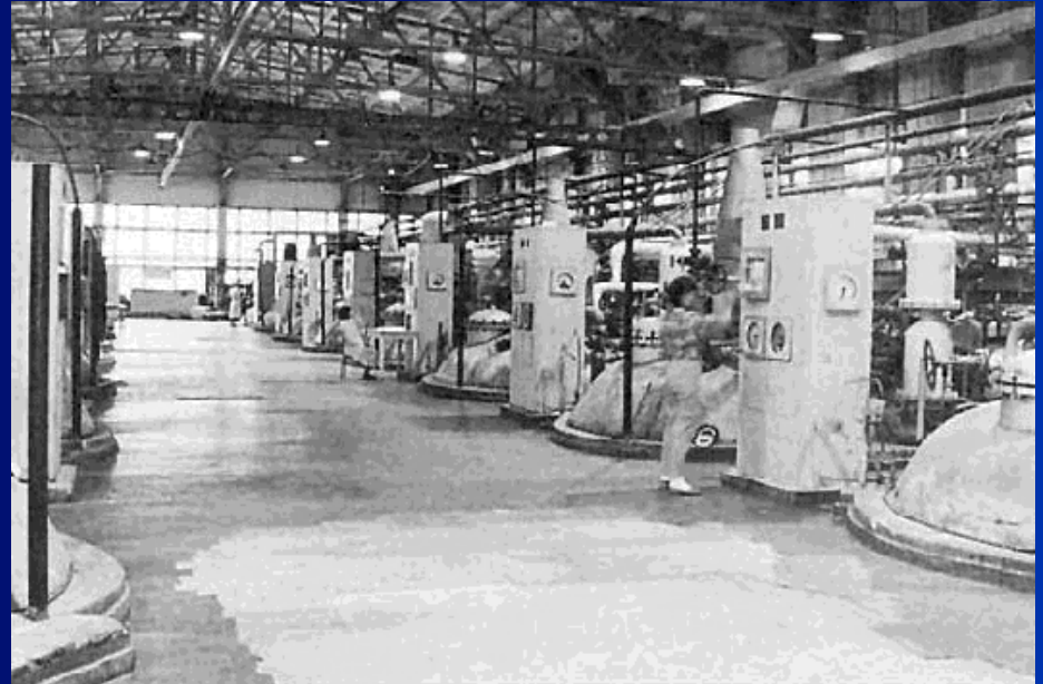
Fermentors in Building 221
