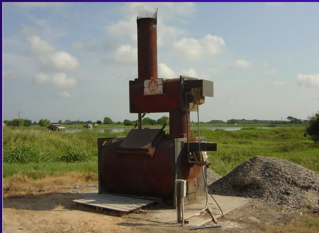
Figure 1. Incinerator for managing poultry carcasses. (NDSU photo)
