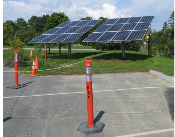
King Arthur Flour electric vehicle charging station
