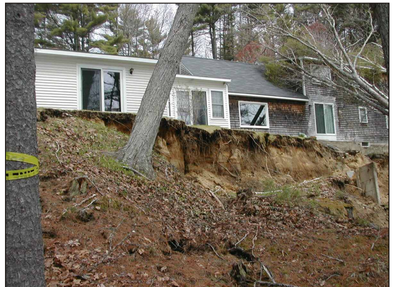
Photo 1. In 2005 a landslide occurred in Wells, Maine along the banks of the Merriland River. The slide destroyed a portion of a walking trail in the Rachel Carson National Wildlife Refuge and removed the backyard of a nearby house. Parts of the house's foundation were left exposed and the house was declared unsafe to inhabit.
