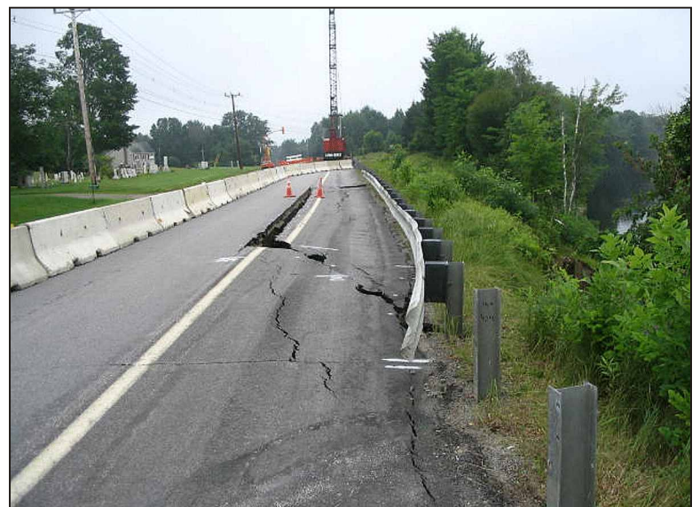
Photo 2. Tension cracks forming and movement along a roadway prior to full slope failure. Downslope forces cause surface layers to stretch. When the tension becomes great enough, a crack forms and some pressure is released. Tension cracks indicate instability and motion along the slope, and are precursors to complete slope failure.
