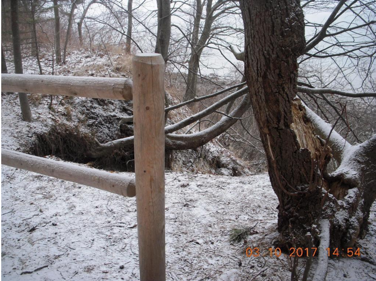
Figure 14. Erosion enhanced through surface water runoff and wave action destabilizes a bluff at Mackworth Island. Land loss next to a trail poses a public safety hazard. Photo by S. M. Dickson.
