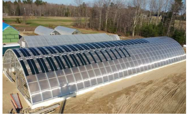
Flexible module application on a greenhouse in Maine Source: Arch Solar
